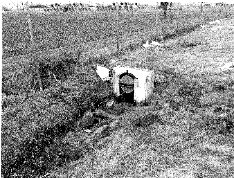
The District replaced a fuel containment spill gate at the maintenance yard to prevent discharge.
